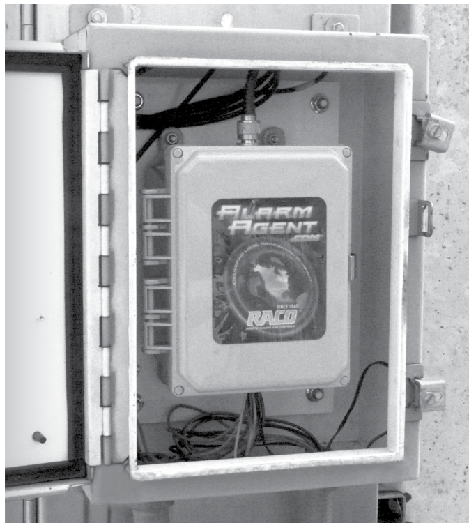
AlarmAgent.com monitors Polk County Utilities's lift stations in a watertight enclosure.
